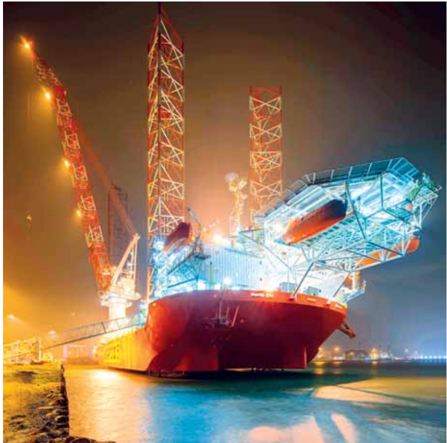
Seafox 5 jacked up 106 times in the installation of monopiles for the DanTysk wind farm off Germany
