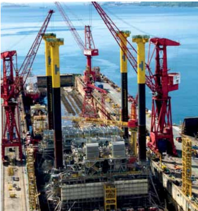
Keppel Subic Shipyard is making good progress on the first complete offshore platform constructed in the Philippines
